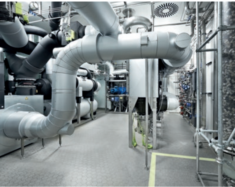
Technical area of a coating system with nitrogen circuit and solvent condensation
